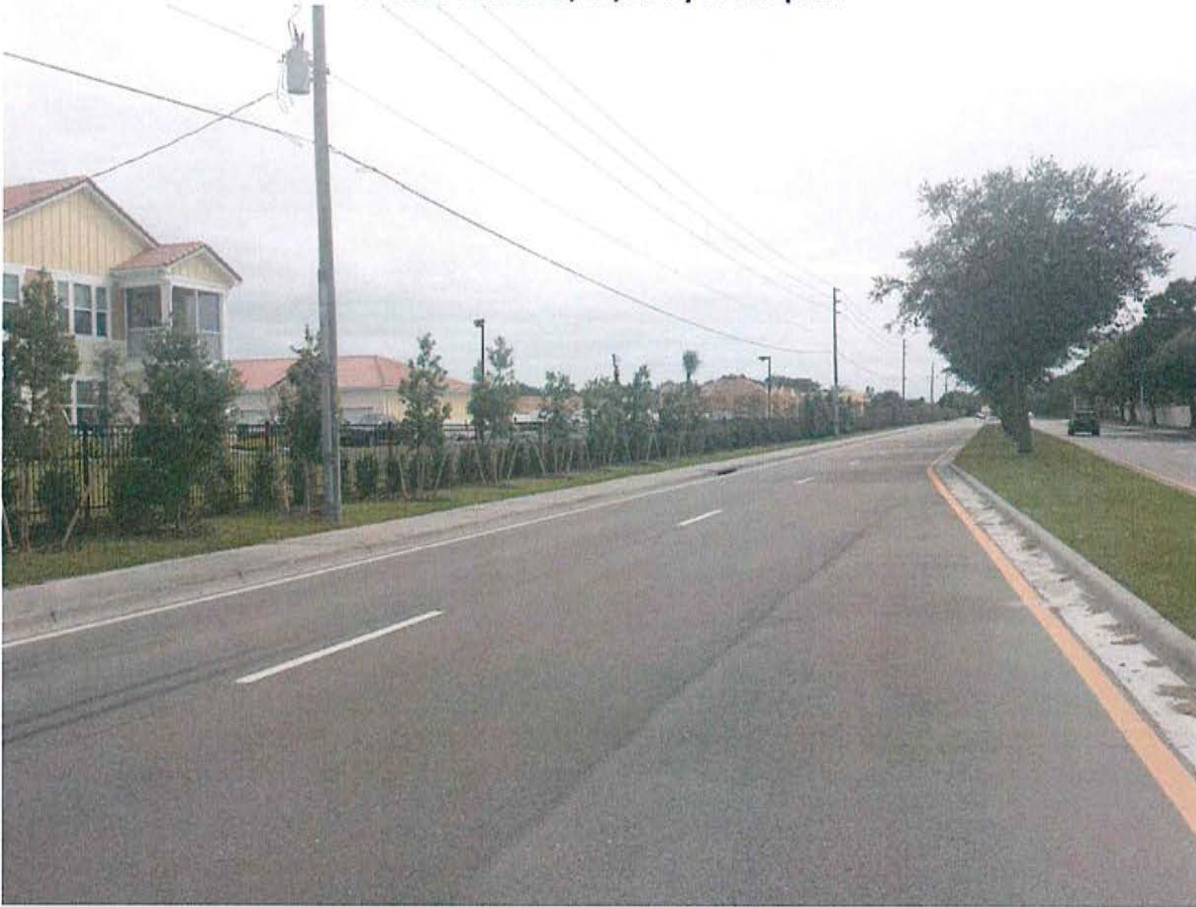
Southerly View along East Side of Cattlemen Rd. Finished units at Left; Construction at Right
